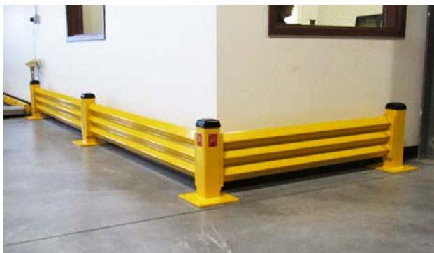
Guarding employees behind drywall
