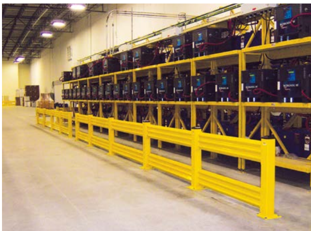
Guarding battery racks
