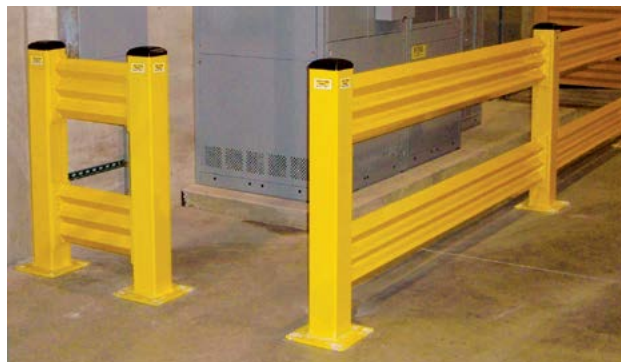
Guarding electrical panels
